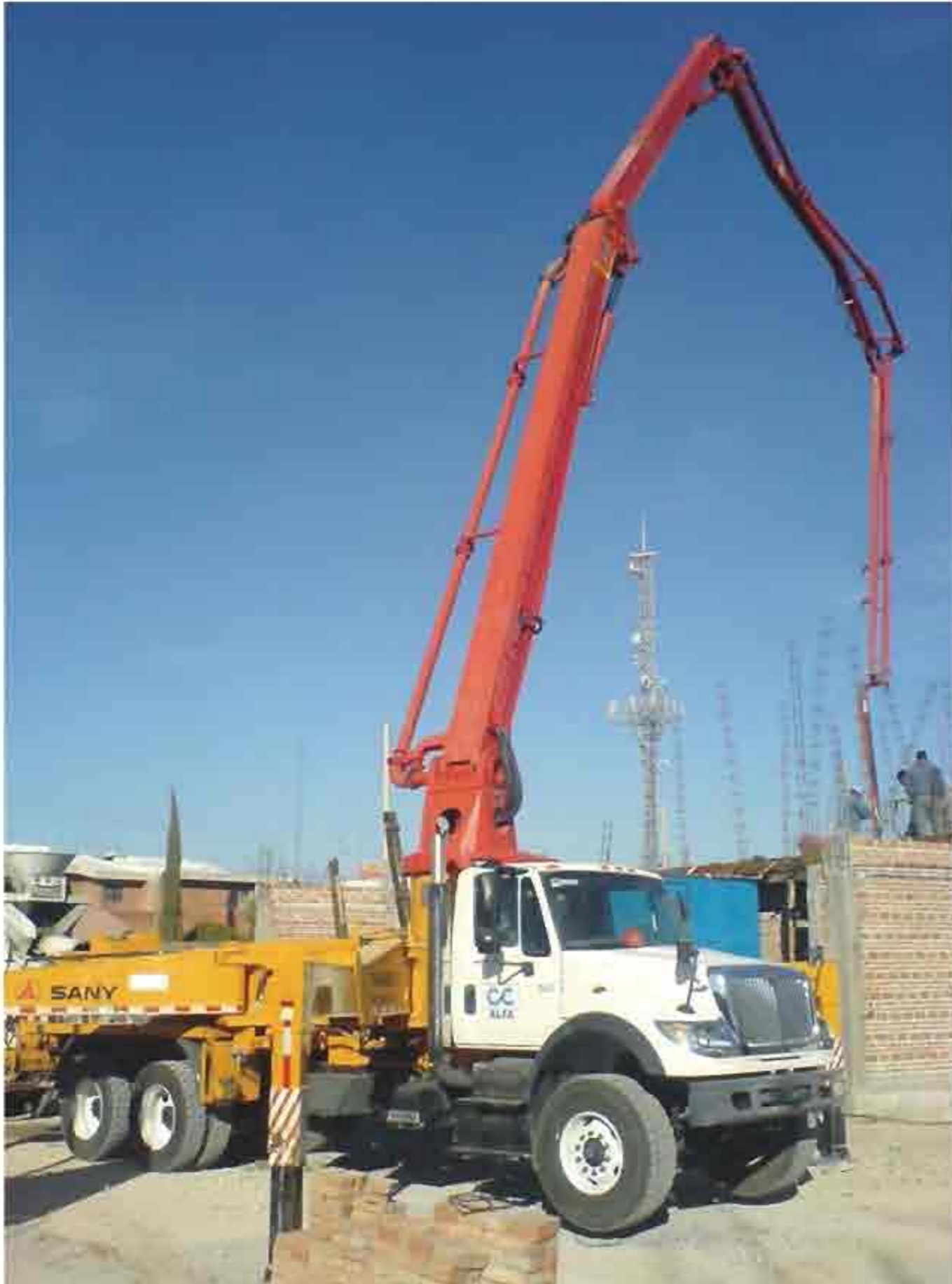
Truck-mounted Concrete Pump at the construction site in the Mexican Torreon Coah Complex.
